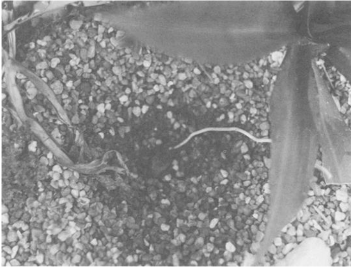
FIG. 4—Cable television service ground investigated by author.
